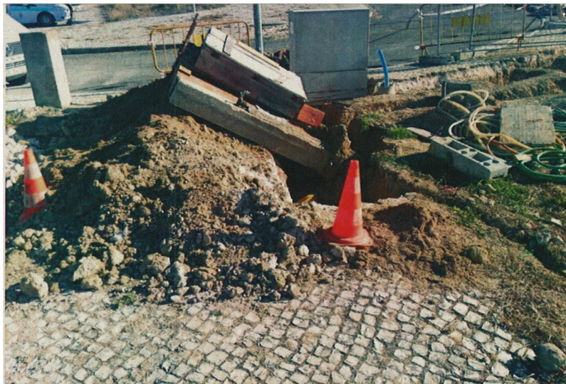
Fig. 1. Death scene demonstrating wall collapse.
