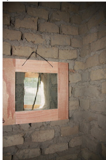
Fig. 2. Installation of GNTs on the (a) exterior of a bedroom window, and (b) the interior window.
