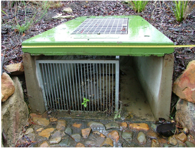
Fig. 1. LitterBank with screened compartment (left) and bypass-channel (right).
