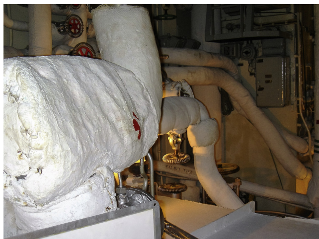
Fig. 1. Asbestos heat insulation in a retired Swedish submarine (photo by Adam Pawełczyk).
