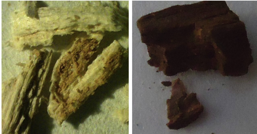
Fig. 1. Wood biodeterioration from white- (on the left) and brown-rot (on the right) attack.
