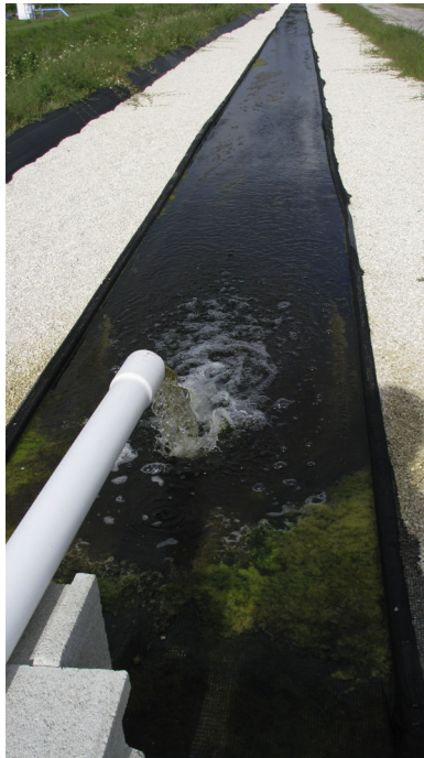
Fig. 1. View of ATS head showing influent pipe and flow-way. Influent poured directly onto the flow-way at 227 \text{ L min}^{-1} . The photo was taken 3 weeks after the influent pump was turned on.
