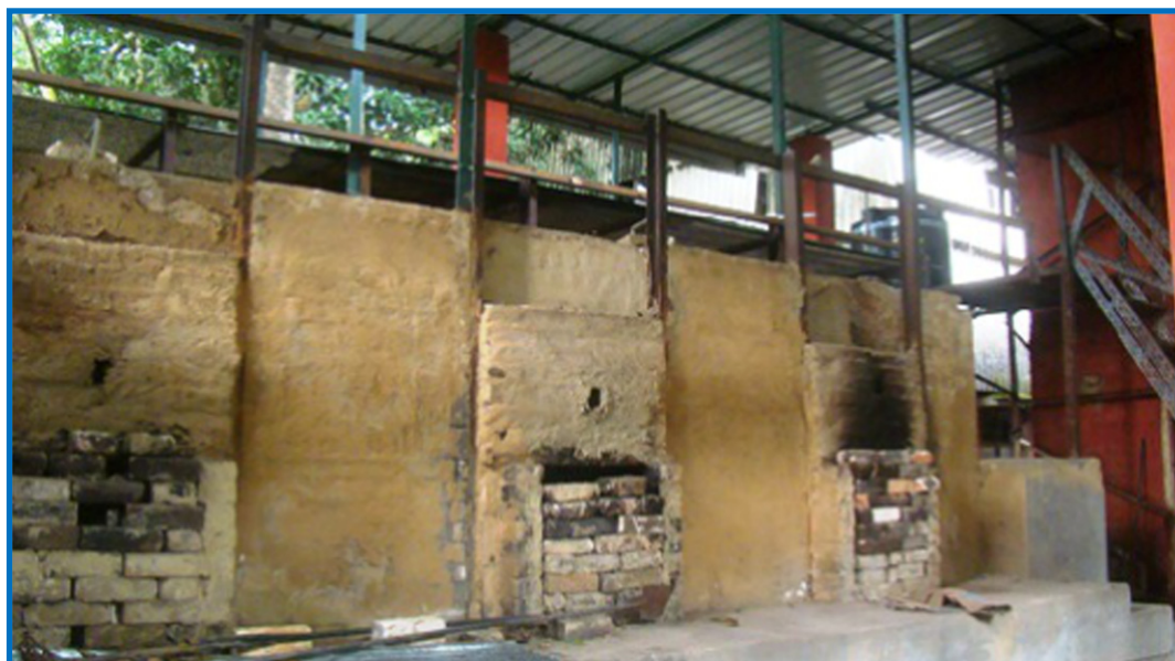
Fig. 2. Coke oven unit used for the study.
