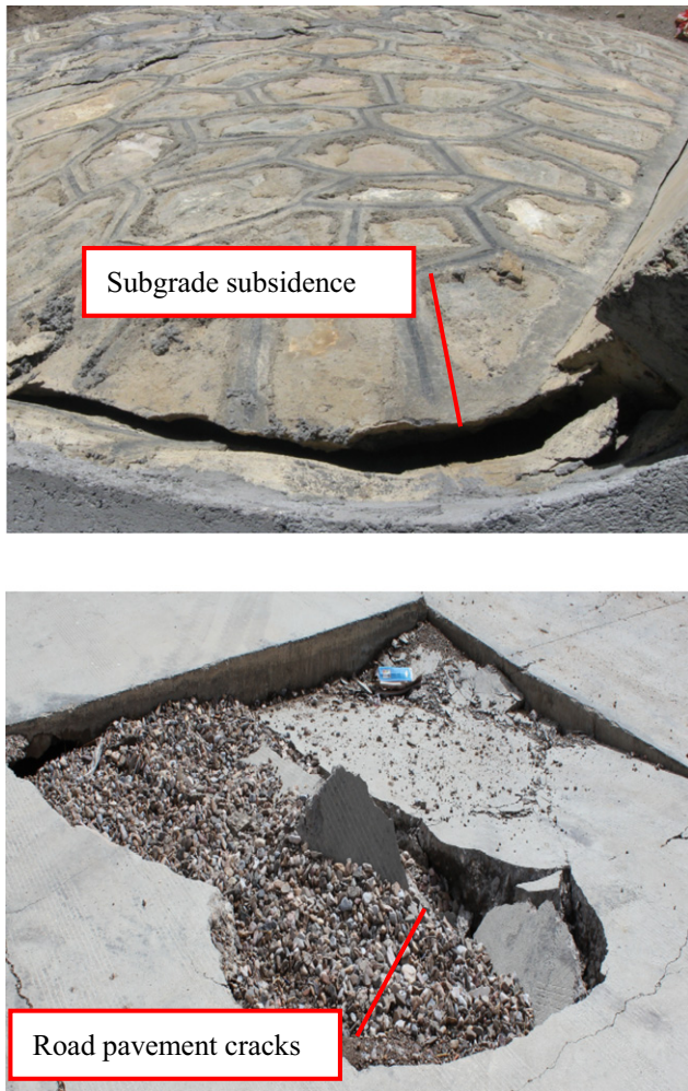
Fig. 1. Damage to engineering structures in the NLCY.
