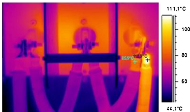
Fig. 2. Parallely cables thermogram in a three-phase installation. Courtesy of ArcelorMittal Tubarão.
