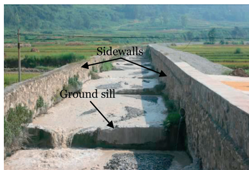
(a) Dongchuan-type drainage channel
