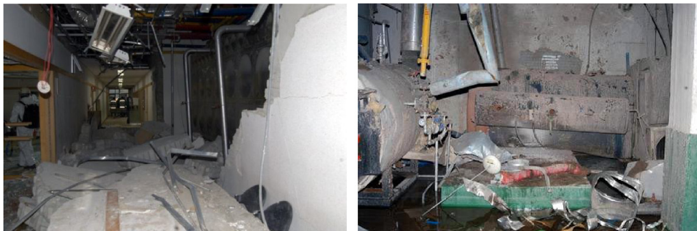
Fig. 1. Photograph of the boiler explosion accident.
