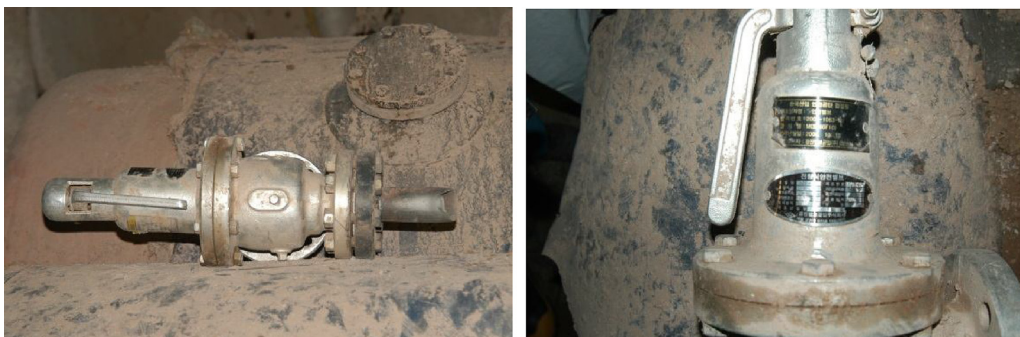
Fig. 2. Photograph of safety valve detached.
