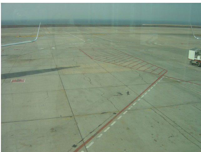
Fig. 1. Cracks in an airport apron – Airport Santa Cruze de Tenerife (photo. K. Falkowski).
