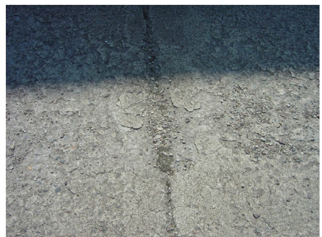
Fig. 2. The loss of the upper layer of concrete after a 20-year usage period (photo. K. Falkowski).
