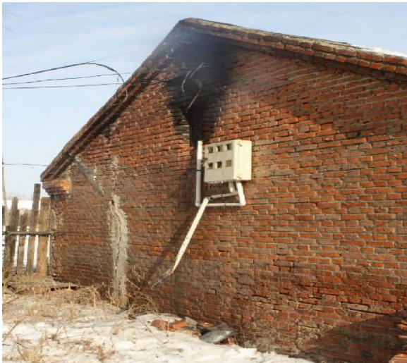
Fig. 1. The rare brick-concrete composite structure houses after the fire. The distribution board and electric meter box were outside the building and damaged in the fire.
