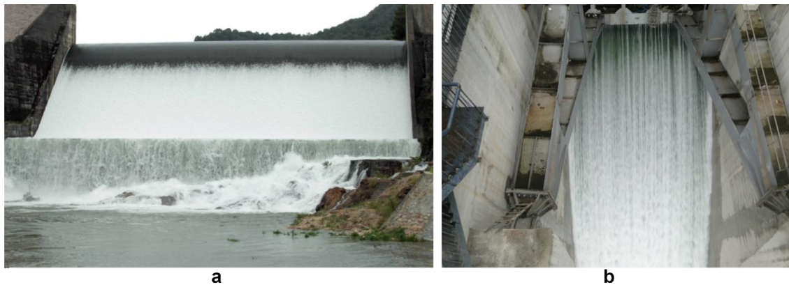
Fig. 1. Free-surface aeration: (a) spillway in Huangtan Dam (Hu et al. 2012); (b) steep chute in Wudu Dam (Imaged by Jun Deng).
