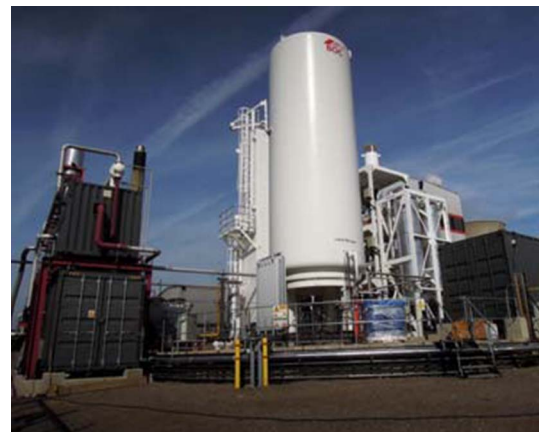
Fig. 1. The first LAES pilot plant (350 kW/2.5 MWh).
