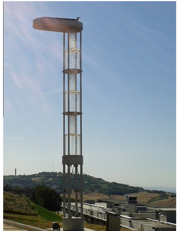
Fig. 1. The UNIVPM prototype of the experimental street lamp powered by renewable sources.
