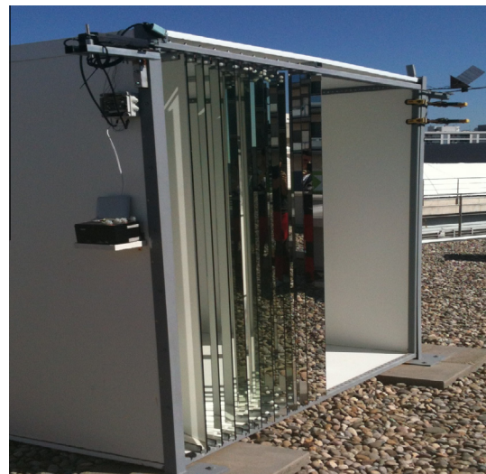
Fig. 1. The reflectors facade: during the installation of the concentrating PV façade at the Applied Energy Research Centre (CREA) at the University of Lleida (Spain). The tracking system is noticed on the left.
