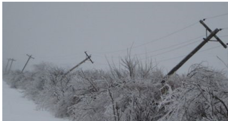
Fig. 2 – Collapse of concrete poles under simultaneous sever wind and snow loads.
