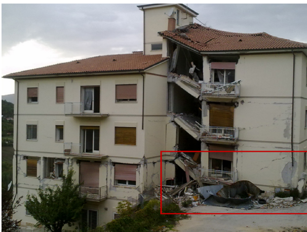
Fig. 1 – Soft storey behaviour due to L' Aquila earthquake (2009).
