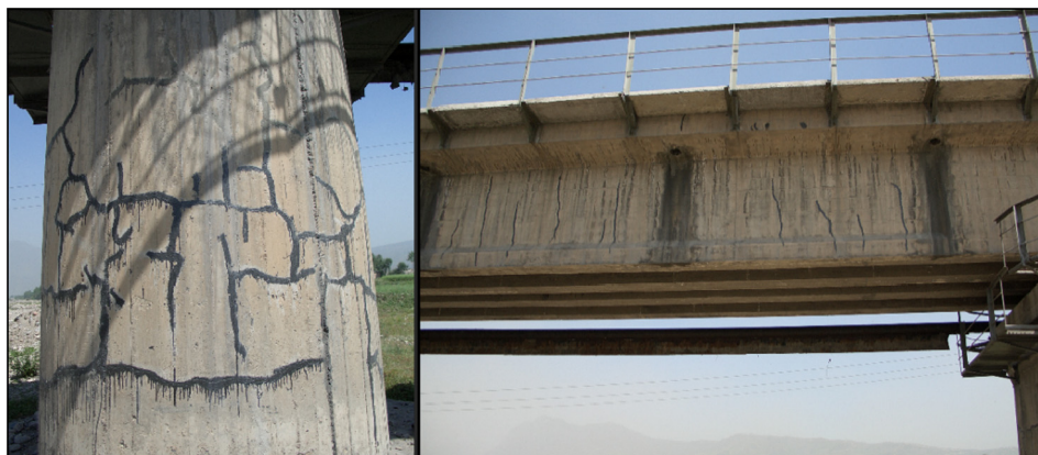
Fig. 1. Concrete damage in low air pressure regions.
