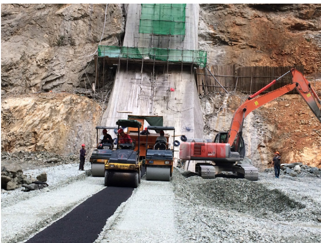
Fig. 1. Asphalt core and transition zone on either side of the core are compacted by three vibratory rollers after being simultaneously placed by a paver.
