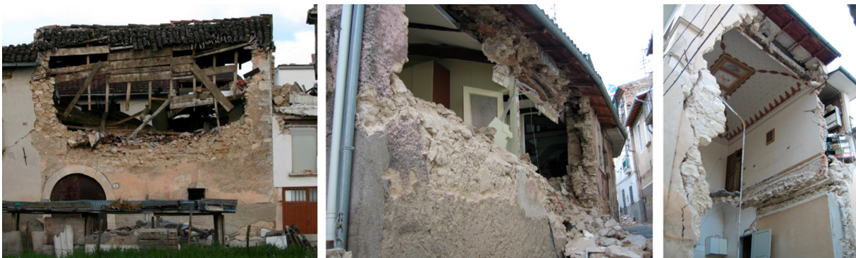
Fig. 2. Examples of common out-of-plane earthquake damage patterns in stone masonry buildings after 2009 L'Aquila earthquake.
