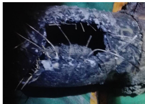
(b) pipeline burst
