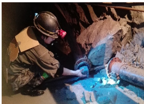
(a) pipeline blockage
