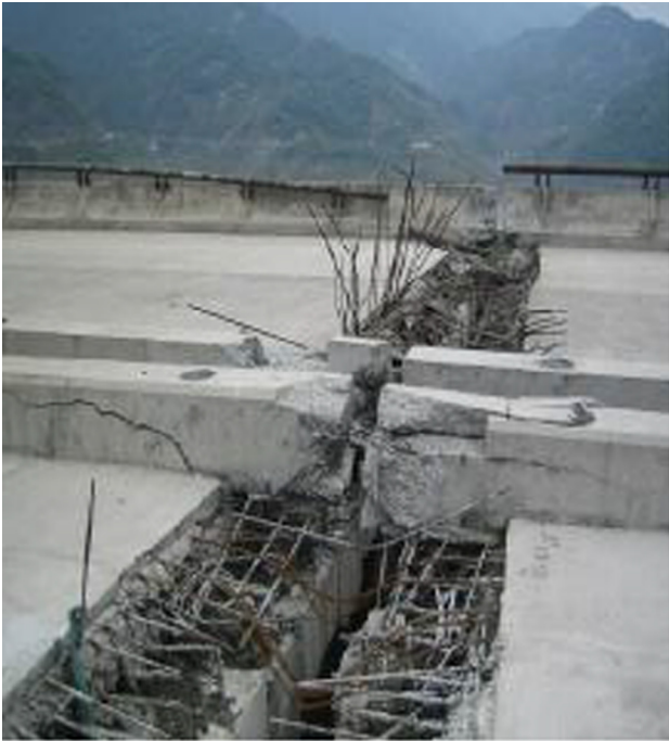
Fig. 1. Collision between girders.
