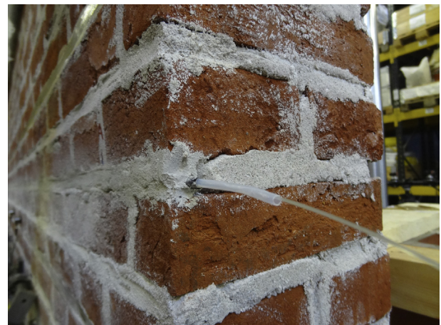
Fig. 1. Ends of the optical fibre (pig tails) at the entrance point in the mortar joint.
