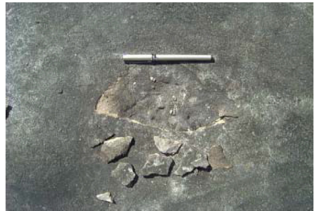
Fig. 2. Scaling at the top layer of the military airbase concrete.
