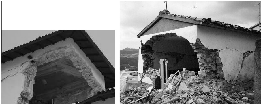
Fig. 2. Examples of an out-of-plane collapse due to poor connection between the RC ring beam and the underlying masonry.
