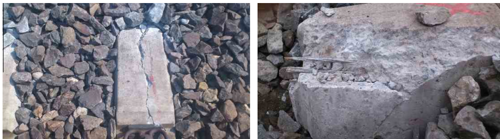
Fig. 1. End cracking of prestressed concrete sleepers.
