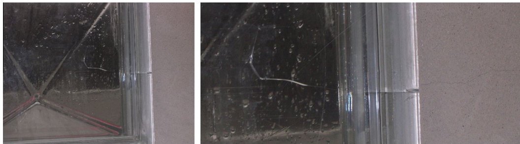
Fig. 2. Damaged glass block and cracked concrete surface.
