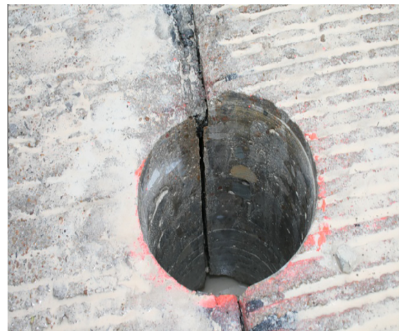
Fig. 1c. Lane separation at longitudinal construction joint.
