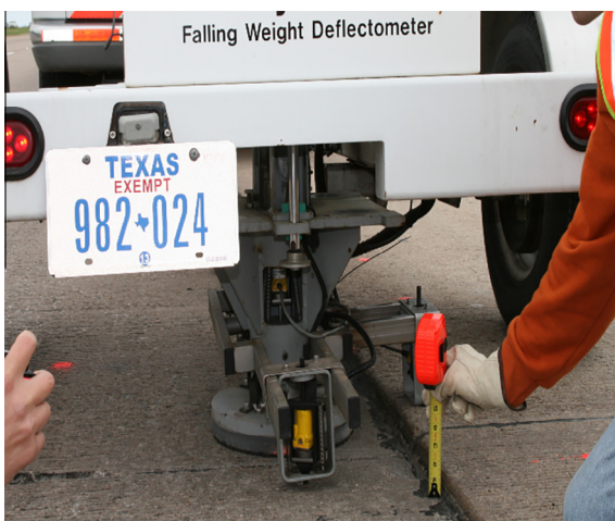
Fig. 1a. Faulting at longitudinal joint.
