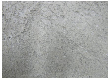
(c) Surface deterioration after 25 cycles of scaling test
