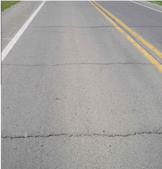
Fig. 1. Thermal cracking in asphalt pavement.
