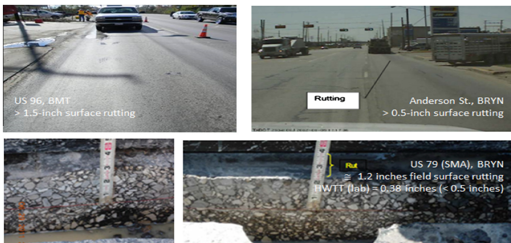
Fig. 1. Examples of premature and surface rutting on some Texas highways.
