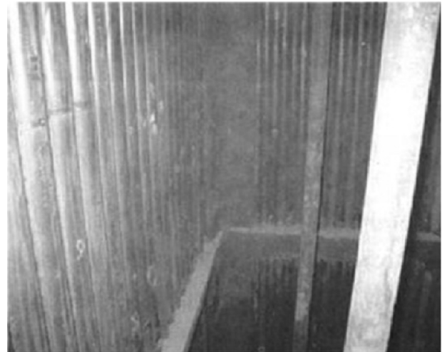
Fig. 1. Anti-wear beams on the water wall.
