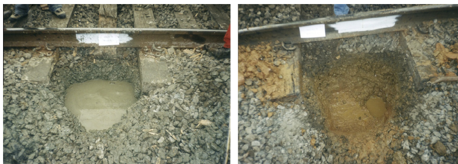
Fig. 2. Water retained in the ballast (left) and state of the platform after water infiltration (right).
