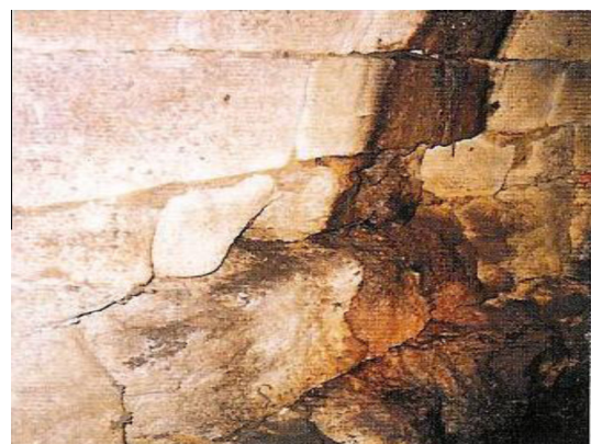
Fig. 2. Stone deterioration due to water infiltration.
