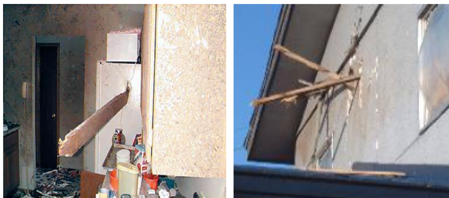
Fig. 2. (L) Windborne missile penetrating a refrigerator in Midwest tornadoes (1999) [16]; (R) windborne missile penetrating a wall [17].
