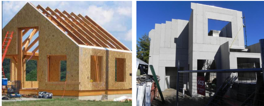
Fig. 1. (L) SIP house with OSB skin [7]; (R) SIP house with fiber cement skin [7].
