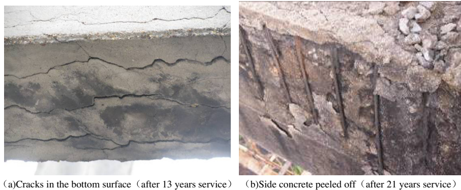
Fig. 1. Photos about deterioration of RC beams.
