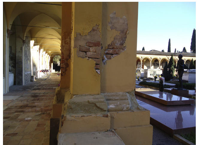
Fig. 1. Persistent problems connected to rising damp in a recently restored part of the Monumental Certosa Cemetery in Bologna, Italy (XIX Cent.). Salt-rich moisture evaporates mainly through the most permeable material (sandstone base) leading to stone decay, and also causes the paint detachment.
