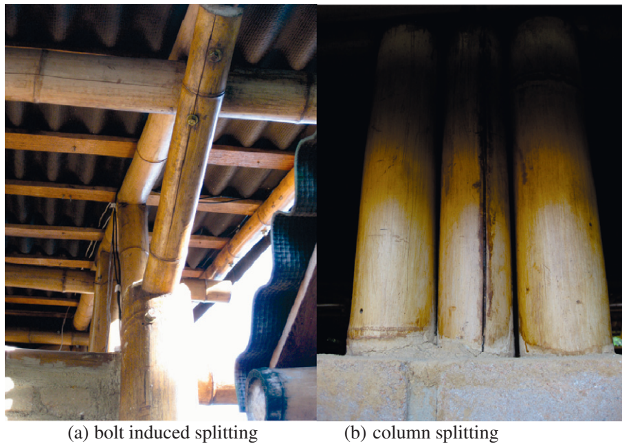
Fig. 1. Bamboo splitting failure observed at Cambury, Sao Paulo, Brazil.
