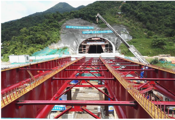
Fig. 1. Photograph of highway bridge girders with corrugated steel webs and concrete filled tubular flanges in construction (Maluan Mountain No.1 Bridge, Shenzhen, China, 2016).
