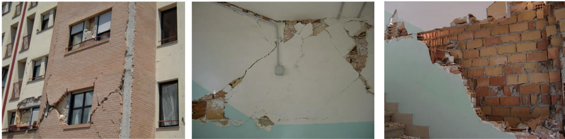
Fig. 1. Damage in the infill masonry walls.
