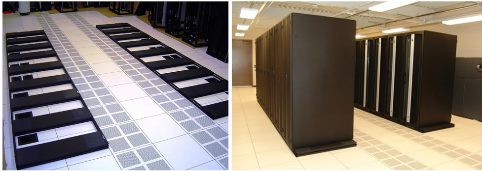
Fig. 1. Multi-unit rolling isolation system array installation at a financial institution data center. Source: [23].
