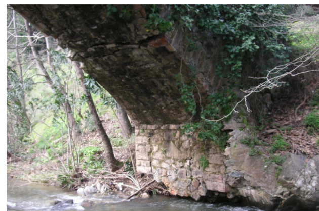
Fig. 3. Kakodiki Bridge: damage in one of the abutments, shown from the upstream side [4,5].
