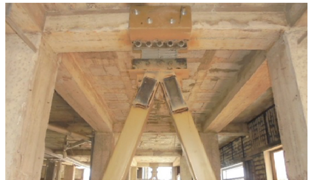
Fig. 3. Installation of a SL for the seismic retrofit of hotel Ceibo Dorado after October 2016 earthquake in Ecuador.
