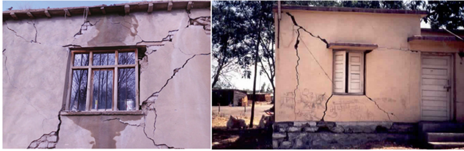
Fig. 1. Damages, in form of cracks, observed in earthen buildings due to hazard-related lateral loading.
