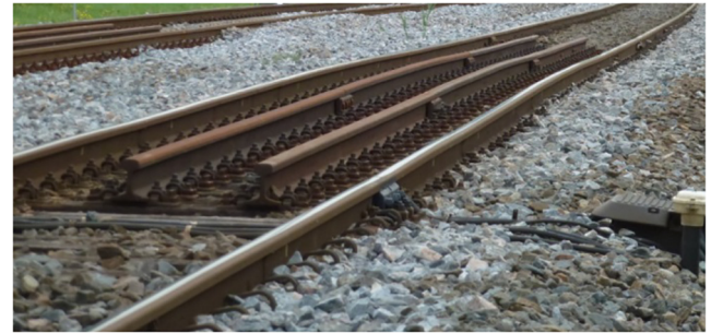
Fig. 3. Transition zone with a large differential settlement, from [18].
