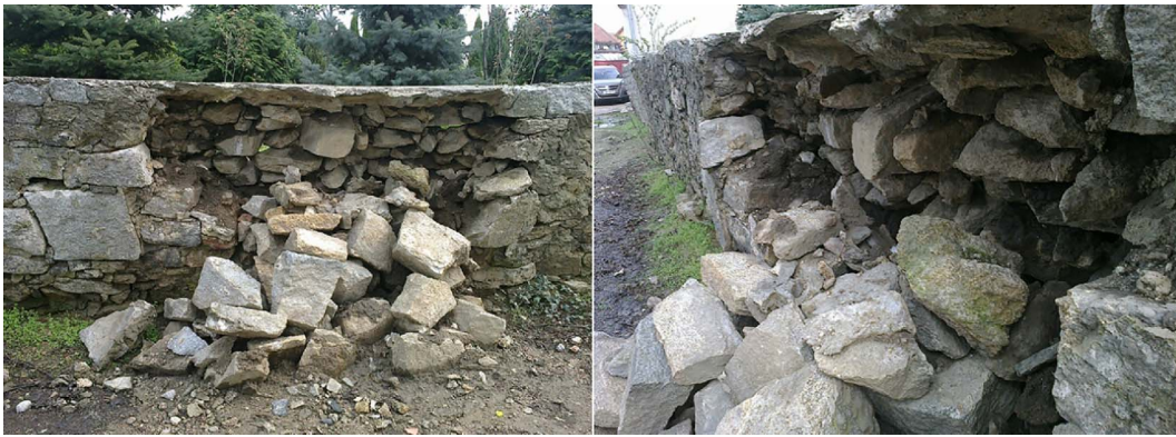
Fig. 1. Free-standing two-layered wall in rural Poland, damaged through the separation of layers.
