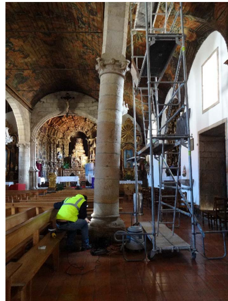
Fig. 2. Photograph of column 2, evidencing its inclination.
