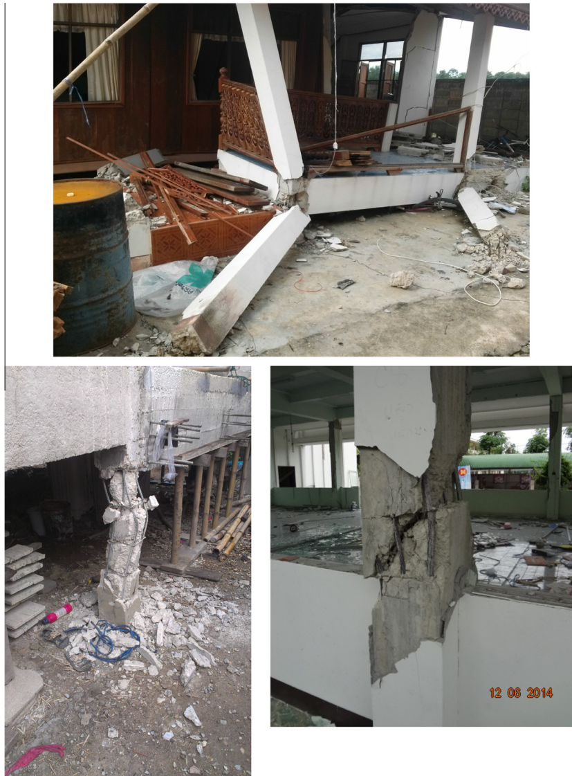
Fig. 1. Failure of RC columns found in 2014 Mae Lao earthquake.
